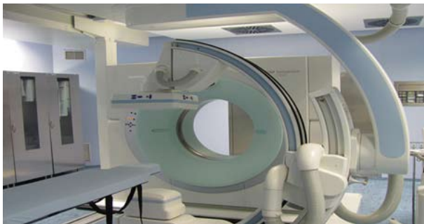
Hybrid Operation Room at the NCI of Bari
